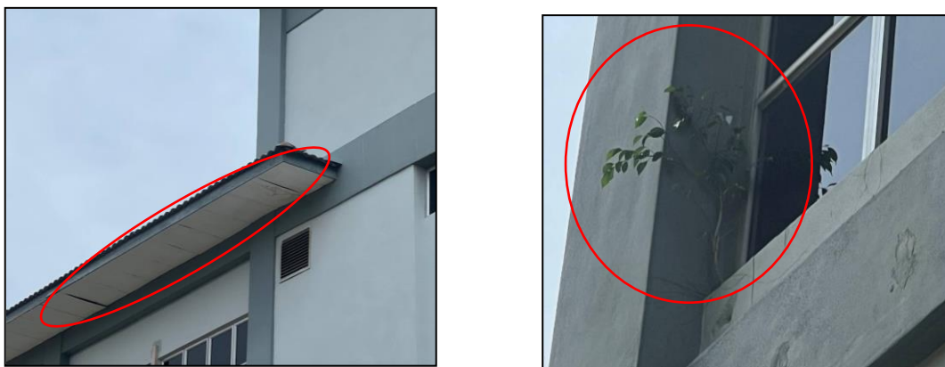
Figure 5: The Dampness And Vegetation Growth Symptom On Fascia Boards Due To Condensation Or High Moisture
