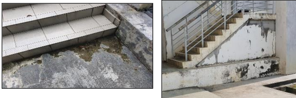
Figure 6: The Standing Water and Mould Growth on Staircases
