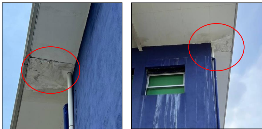
Figure 4: The Dampness Symptom Due to Clogged Downpipes
