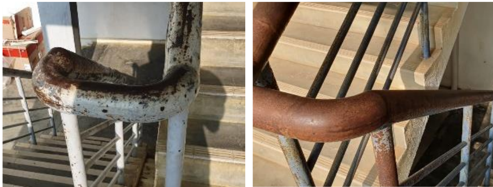
Figure 7: Corrosion of Handrails Due to Dampness
