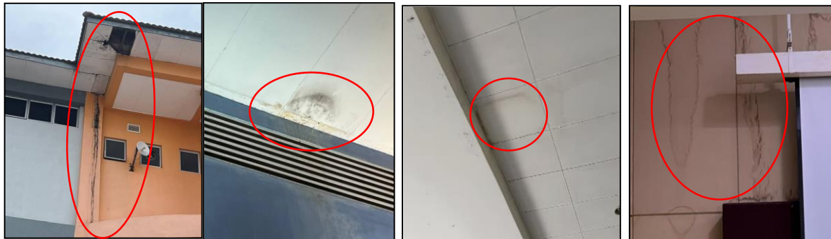
Figure 3: The Dampness Symptoms Caused by Roof Leakage.
