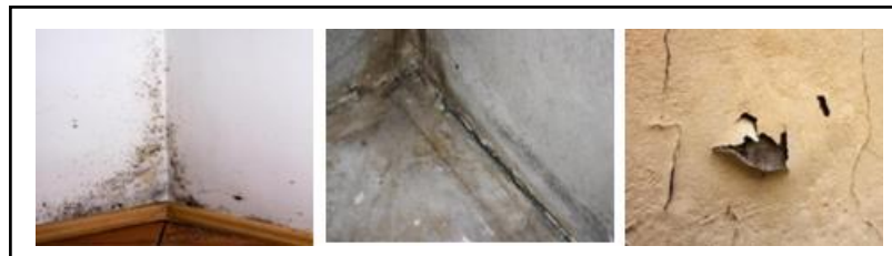
Figure 2: The Building Defects Associated With Dampness
